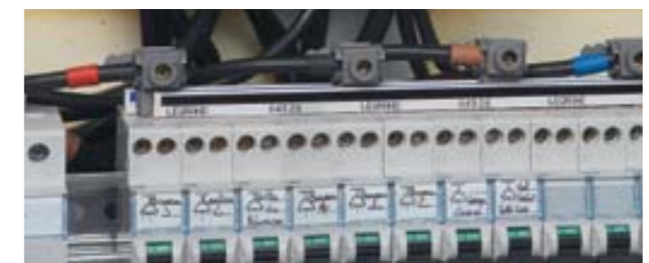
^ Distribution via supply busbars
